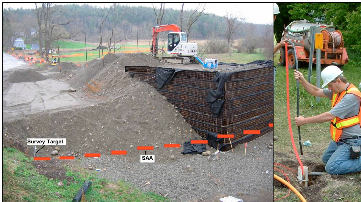
Figure 3: Left: 2D Deformation Monitoring Near a Bridge Abutment Right: Installation of an SAA for 3D monitoring
